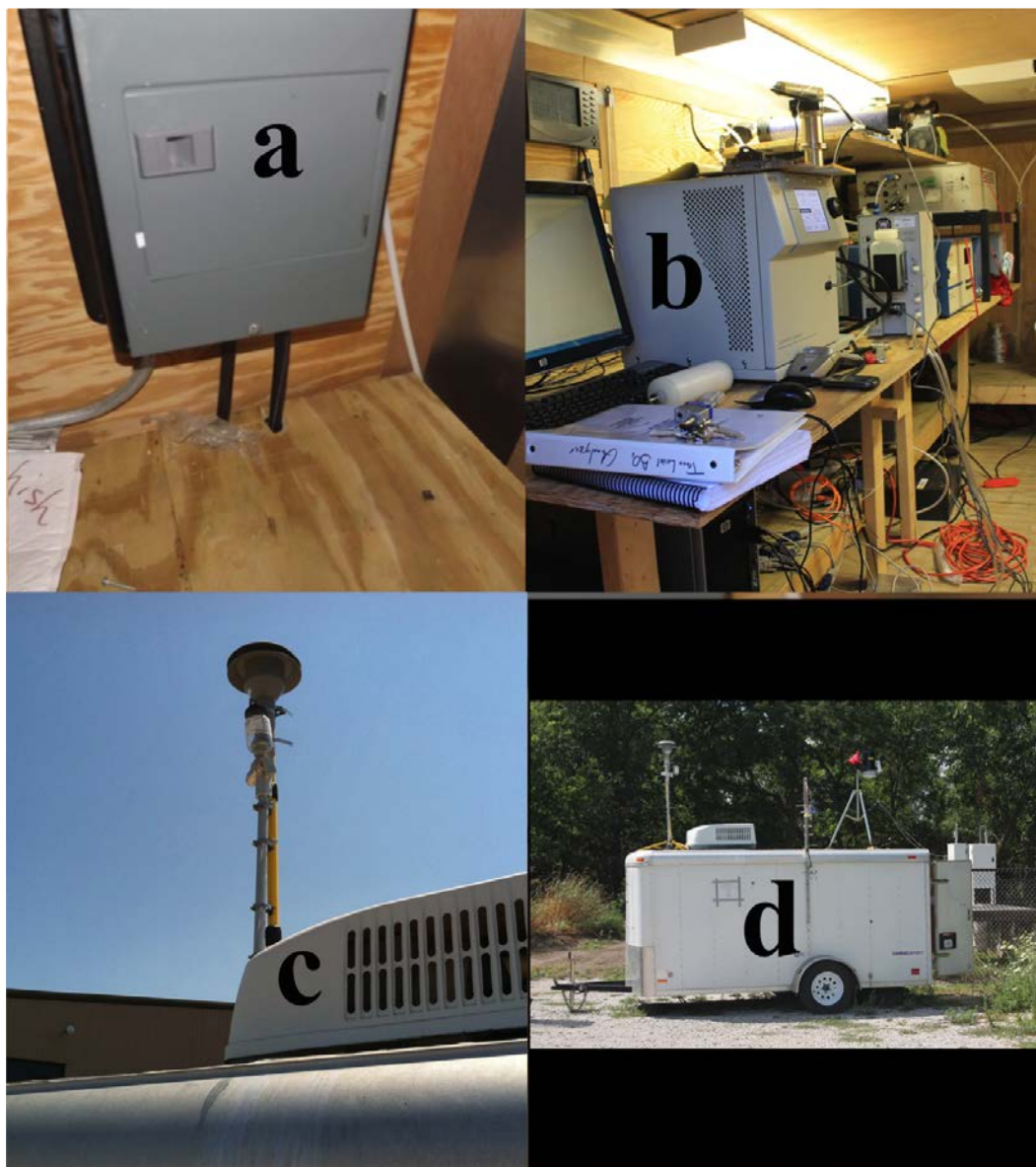
Figure 3.9: The electrical setup in Figure 3.9a allows for two 15A circuits to feed one electrical panel. Circuits with 30A capacity are often not available in remote field locations, where multiple circuits with a lower amperage may exist. This setup allows some versatility in getting enough power to run the instruments in the trailer. Figure 3.9b shows the capacity of the trailer to house gas and particle instrumentation with appropriate aerosol inlets for minimized particle loss and the use of inert materials for gas inlet lines. Figure 3.9c shows the inlet borrowed from the Peters lab, it allows isokinetic, real time sampling of PM_{2.5} . The inline drier and extended mast are additions by the Stanier lab to ensure sampling of dry aerosol and representative sampling of the atmosphere by minimizing disturbance of the sample stream by the trailer. Figure 3.9d shows the full trailer setup used during the power plant field campaign. The front features a weather station with a wifi hotspot to sync data to Dropbox.
